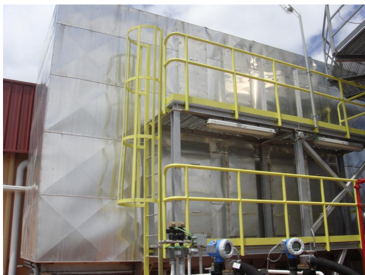
External view of the SCR system in Ceuta
