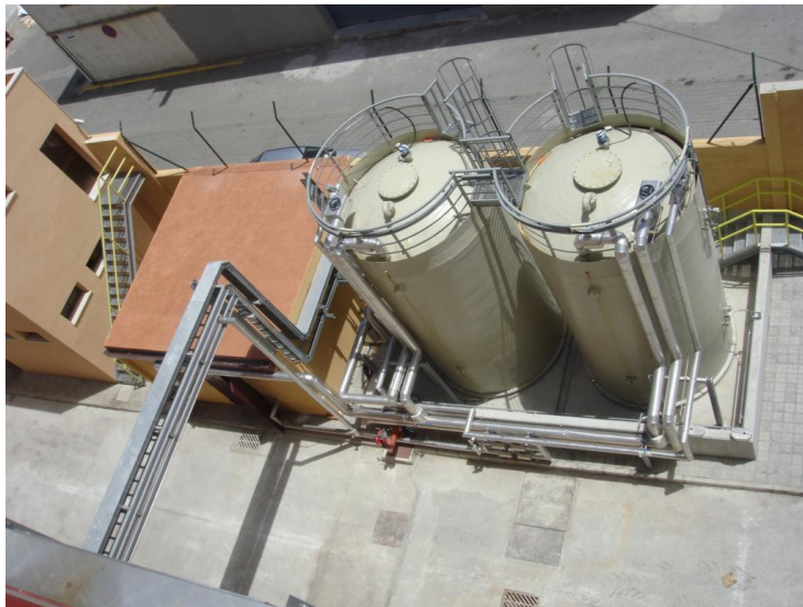
Aerial view of the SCR system's urea tanks in Ceuta
